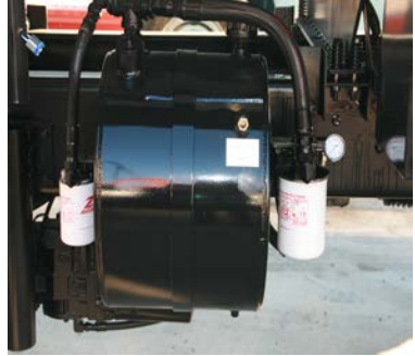
Hydraulic Reservoir and Filter
