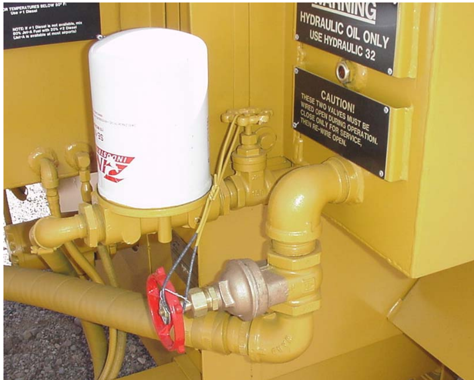
Figure 3-6. Hydraulic Reservoir Gate Valves
