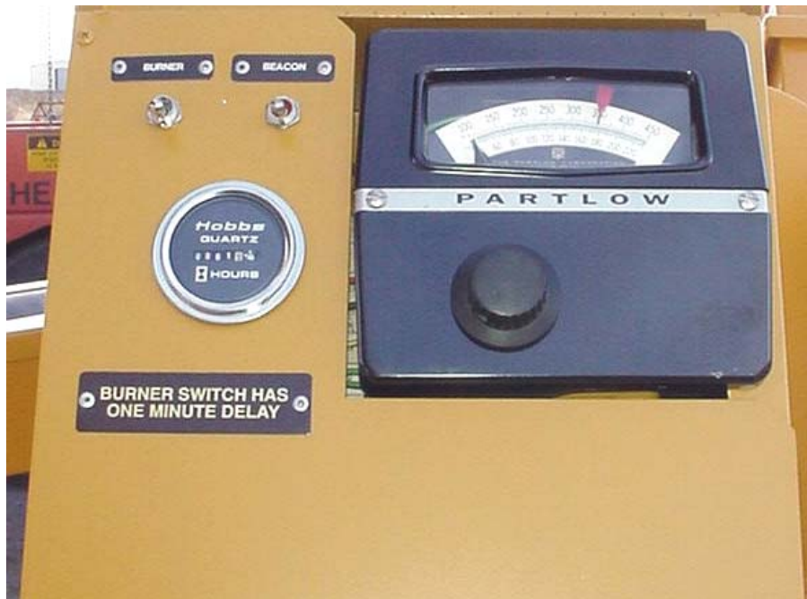
Figure 1-15. Temperature Control Panel
