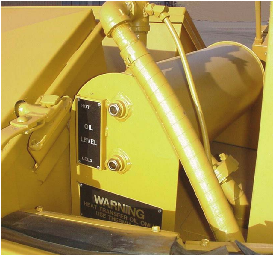
Figure 1-14. Hot-Oil Expansion Tank and Sight Glass
