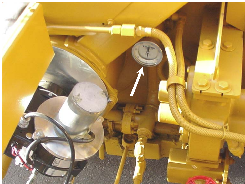
Figure 1-16. Hot-Oil System Temperature Gauge
