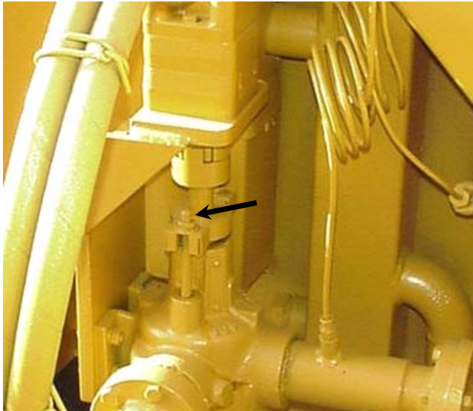
Figure 5-6. Hot-Oil Pump Retainer Bolt
