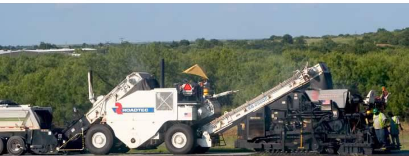
Use of the Shuttle Buggy® material transfer vehicle with the gravity-fed Spray Paver allows crews to pave without stopping and produces smooth, segregation-free pavements in record time.
